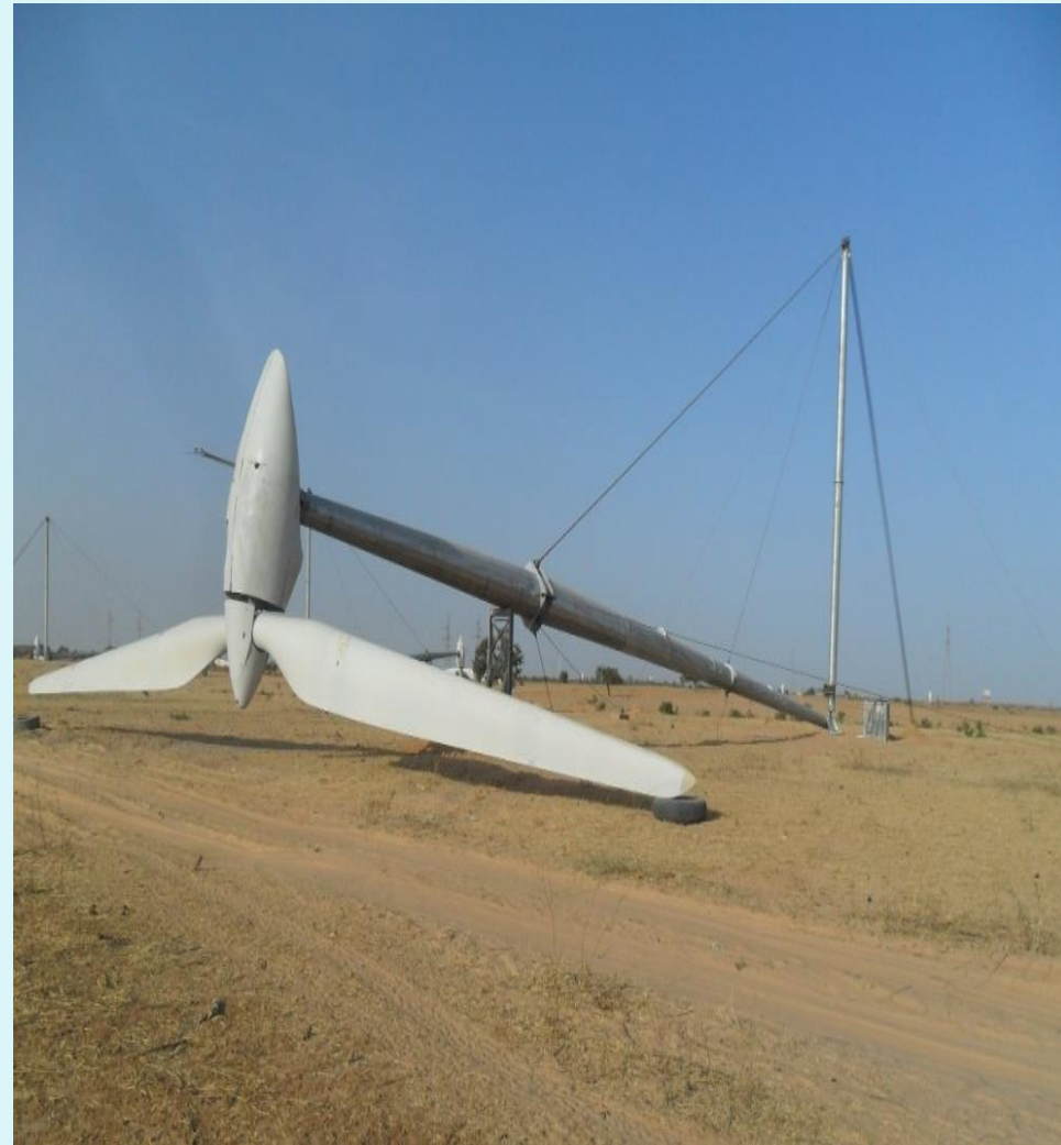
One of the 37 No 275kW Wind to Electricity Machines for the 10 MW Katsina Wind Farm
